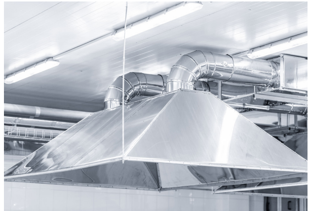
Figure 12. A large industrial vent hood.
